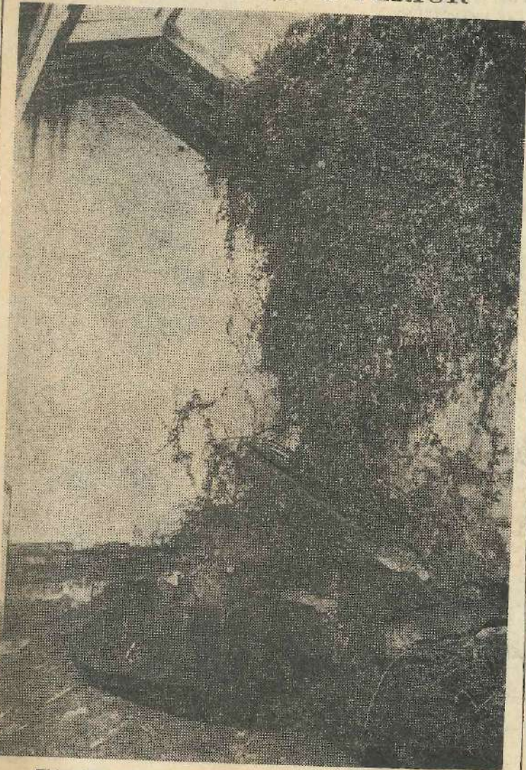
This picture shows one of the baths in White Wells, a creeper growing up the wall and rafters exposed in the ceiling. Repairs are now being carried out.
