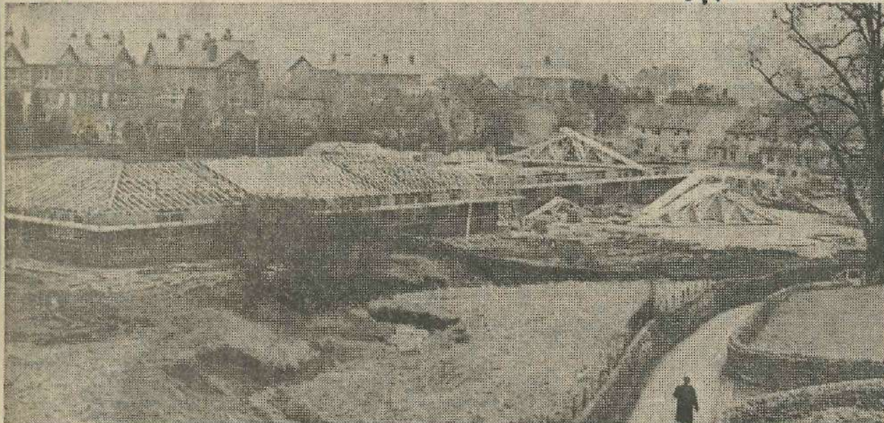
Work was well under way on construction of Addingham's new Middle School on land at the junction of Back Beck Lane and Bolton Road when the picture above was taken in April. The new, $440,000 school will accommodate 260
